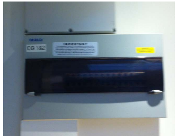
Level 1 & 2 Consumer Unit in 1 st floor Hall cupboard
