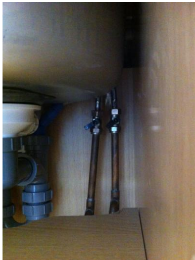
Shut-Off Valves under Each Sink
