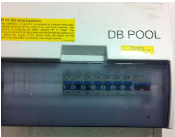
Pool Consumer Unit in Pool House plant room
